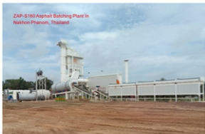
ZAP-S160 Asphalt Batching Plant in Pichuph Khiri Khan, Thailand
